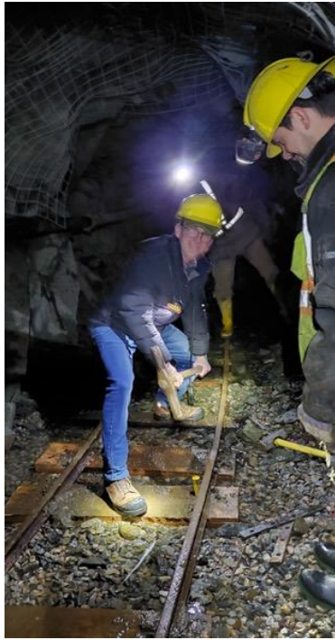
Photo of CEO Christopher Anderson hammering in the “Golden Spike” connecting the new underground rail with the Kenville 257 Level rail line.
