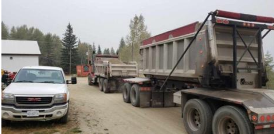
Photo of truck arriving at Kenville Mine carrying crushed gravel for culvert bedding
