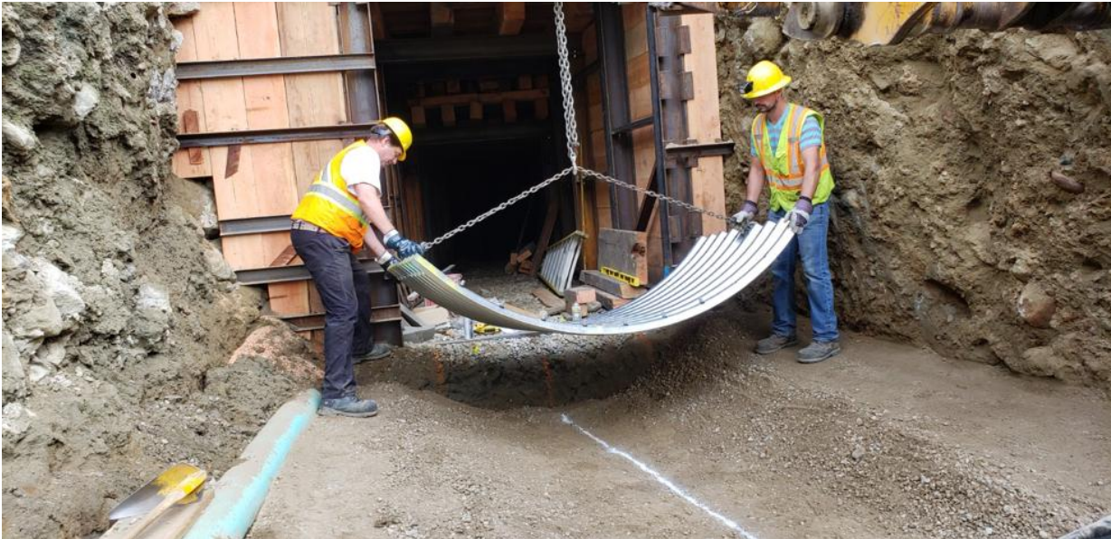
Photo of first section of culvert being placed outside of Kenville 257 Portal.
